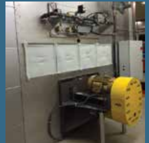
FILTERED INTAKE AIR
