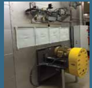
FILTERED INTAKE AIR
