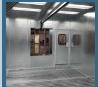
Raised & Grated Containment Floor
